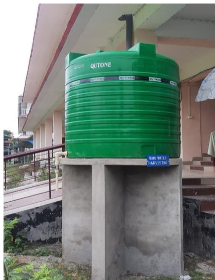
Photo 3: Rain Water Harvesting Unit
